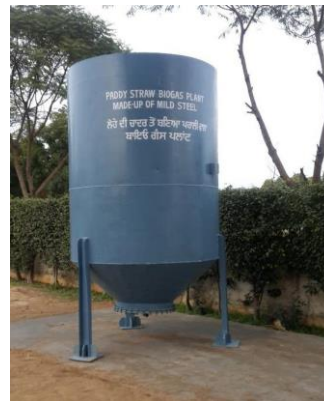
Fig 2: Paddy straw based biogas plant made up of mild steel.
