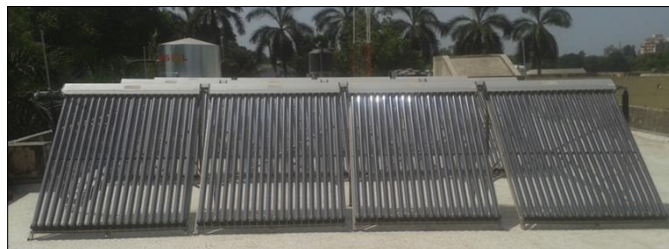
Fig 4: Solar hot water heating system with ETC-HP
