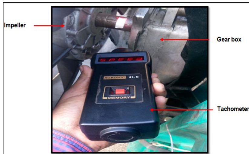
Plate 2: Measurement of blower speed
